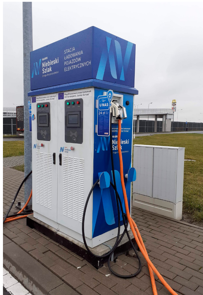
Charging station in Brwinów at A2 motorway
